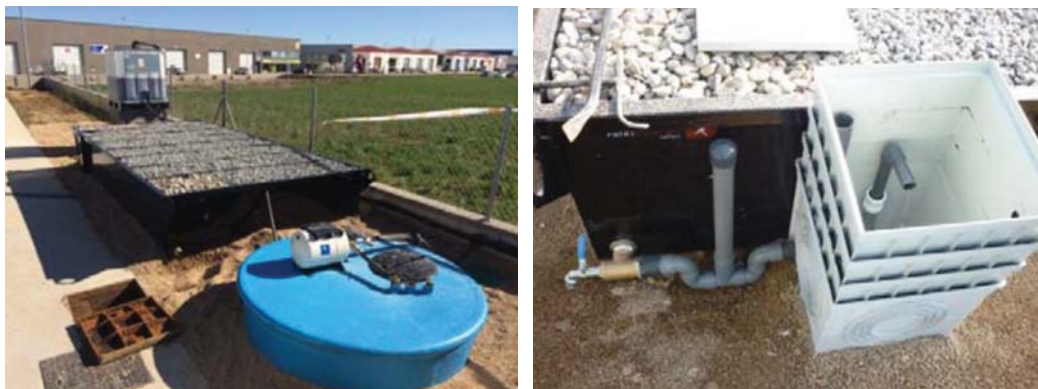
Figure 21.4 Pilot HFCW container and outlet device.
